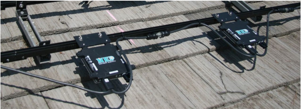
NEP BDM-300 Inverters daisy chained in a branch circuit
